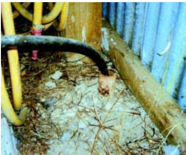
Poor well head protection.
