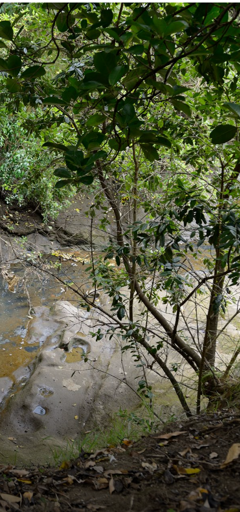
► Stormwater pipe at Cox's Bay Reserve, Auckland.
