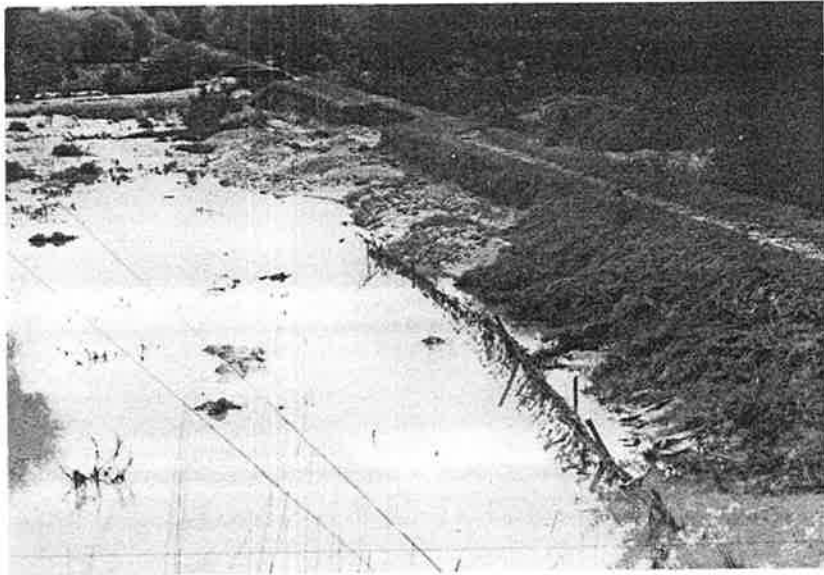
Stopbank (true right bank) immediately upstream from Saleyards Bridge (Opihi River) demonstrating process of stopbank failure. Flow overtopping the bank erode the stopbank from the top back towards the river side of the bank (mid photo) until eventually the bank is totally breached (top left photo).
