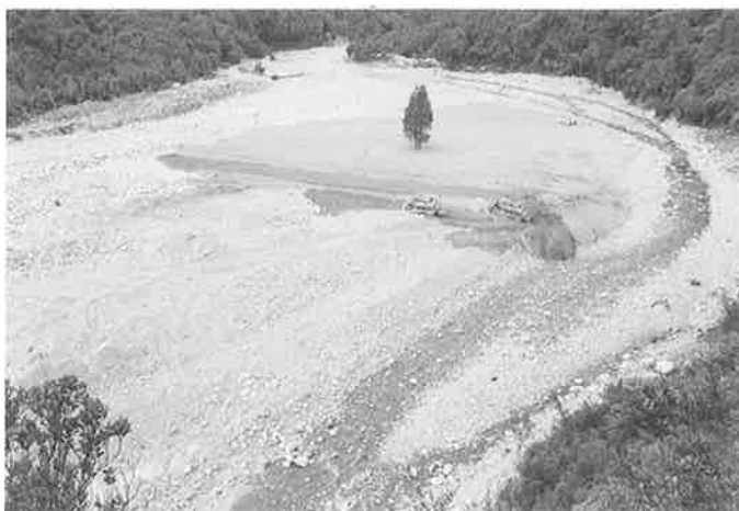
FIGURE 9. The Big Hohonu River Diversion, March 1988. Stock-piled topsoil is being re-distributed over the floodplain. The stream tends to the true right of the channel.
