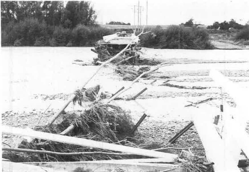
Many bridges throughout Strathallan and Waimate Counties sustained major damage. Brasells Bridge built in the early 1900s was extensively damaged.
