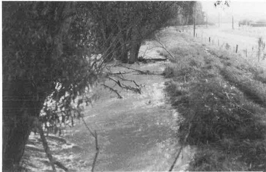
Hinds River within 300mm from top of stopbank between Poplar Road and Surveyors Road (Black Bridge).
