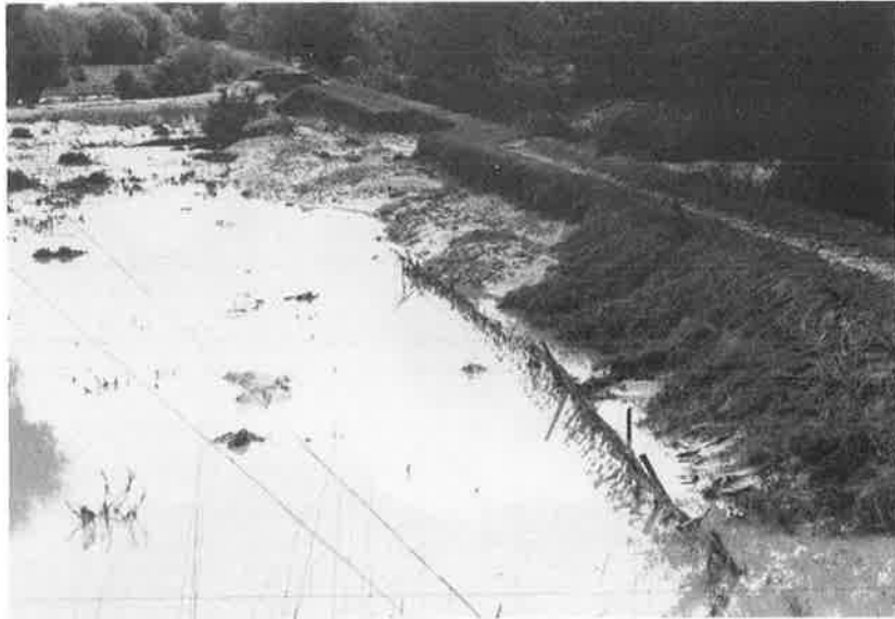
Stopbank (true right bank) immediately upstream from Saleyards Bridge (Opihi River) demonstrating process of stopbank failure. Flow overtopping the bank erode the stopbank from the top back towards the river side of the bank (mid photo) until eventually the bank is totally breached (top left photo).
