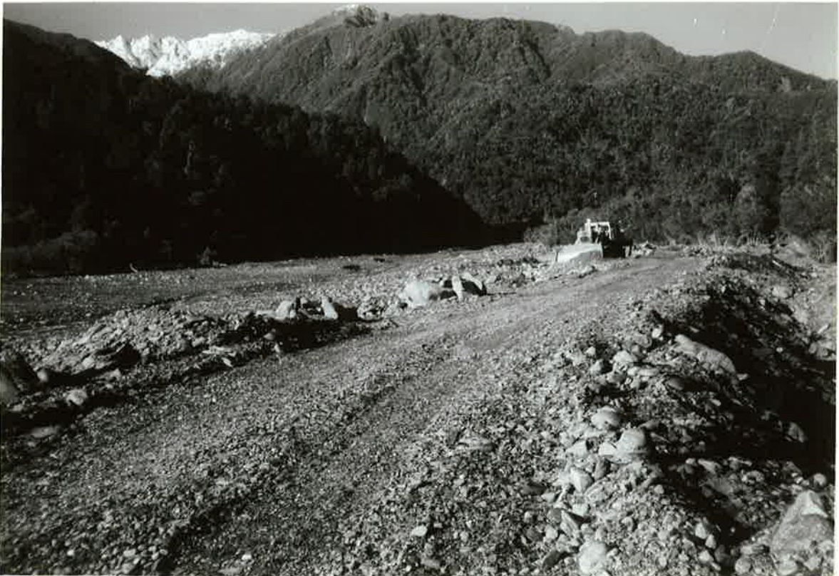
FIGURE 32. Flood prone Havelock Creek, and the bulldozer used to prevent flooding of S.H.6 bridge. No fish were collected from this stream.
