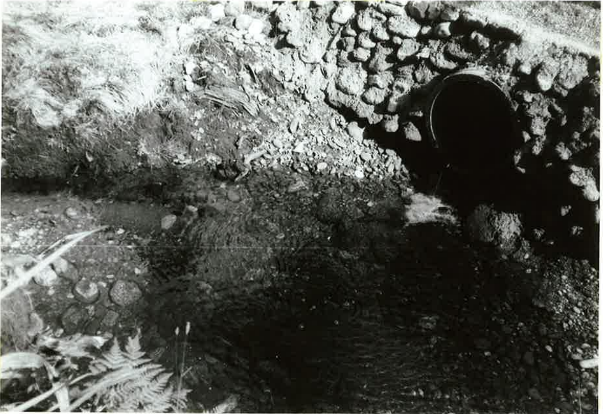
FIGURE 31. Culvert on a tributary of Pita Creek at S.H.6. Note the free fall of water. This barrier prevented upstream migration of three species of fish.
