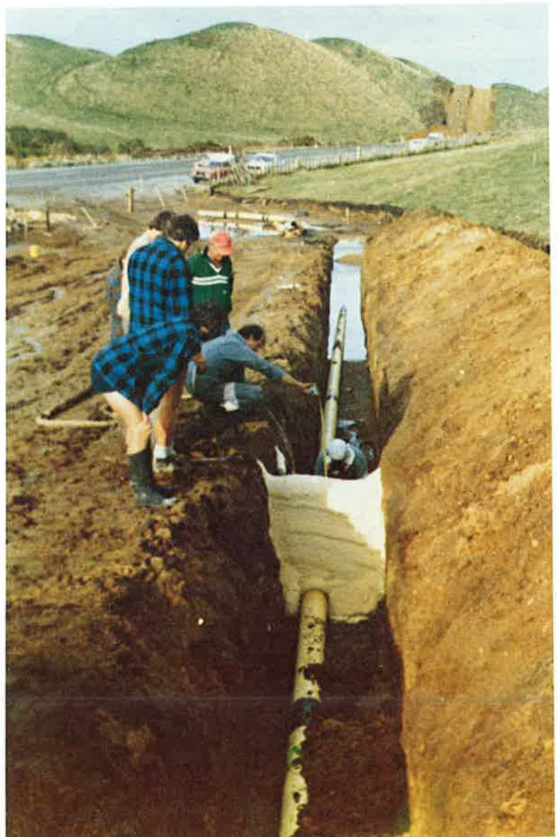
Figure 5: Kinleith—Kawerau natural gas line, 1982. Foam breakers can be used to stop water flowing down the trench and to support backfill material.
