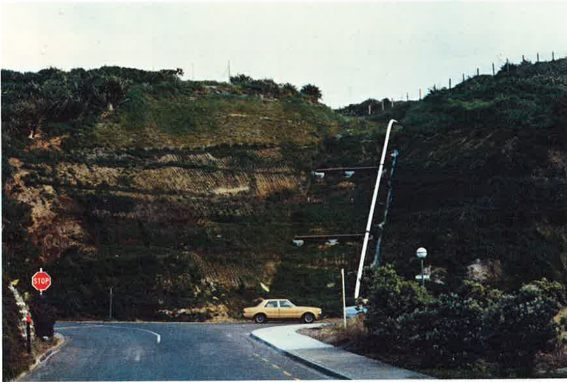
Figure 8: Port loading line, New Plymouth, 1983. This face was difficult to reinstate. The top section, which is sand, was covered with plastic mesh and a wood fibre mulch and then seeded. The lower section was hydroseeded. The bench drains were planted with flax.
