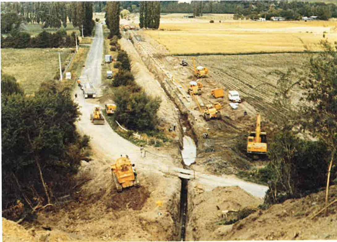
Figure 4: A section of the Hawkes Bay natural gas line being laid near Ashhurst, 1983. Note the problems of using a restricted right-of-way through areas of cropping. Vehicles damage the topsoil by using it to gain access to the line.
