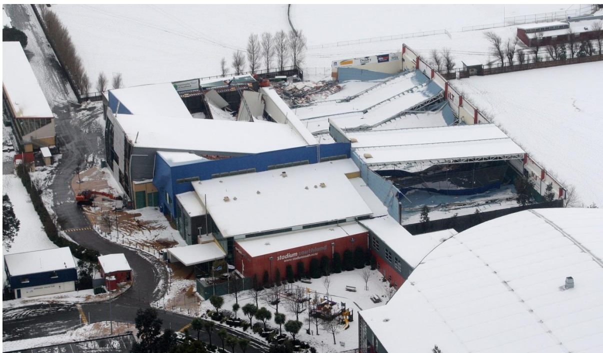
Figure 10-1: The roof of the Southland Stadium in Invercargill collapses under a blanket of heavy wet snow. 18 September, 2010 (photo used with permission of Fairfax Media).
